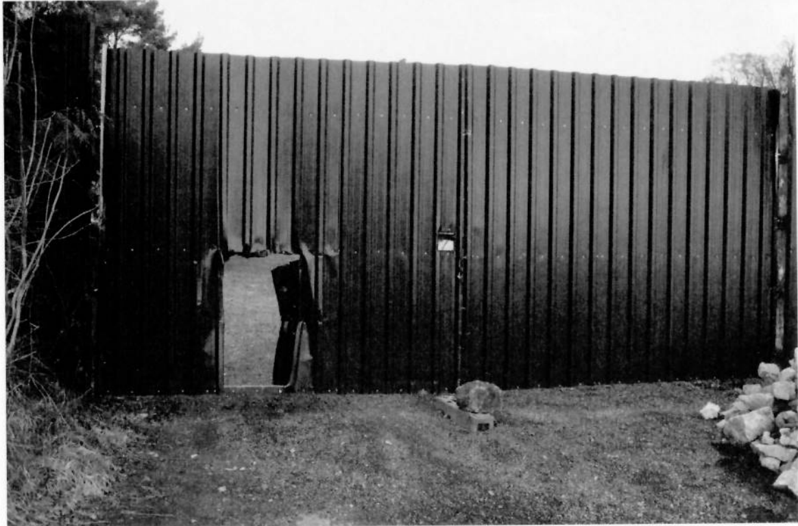
Poorly executed and utilitarian metal gates more akin to a junk yard.
